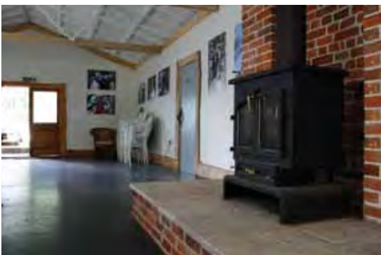
Wood burning stove heating a classroom at New Forest Outdoor Centre, near Minstead.
