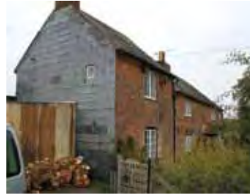
Slate is quite adaptable, shown here used vertically. It is also commonly used on shallow roofs.
