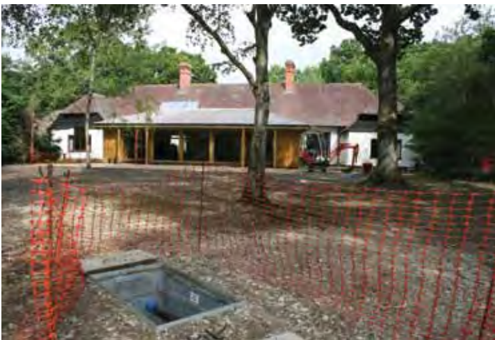
Ground source heat pump installation at Ferny Crofts Scout Activity Centre, near Beaulieu.
